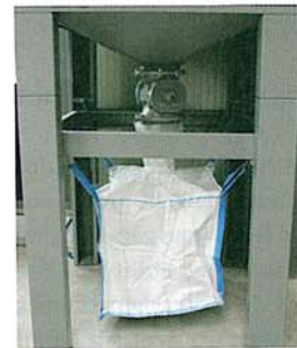
The rotary gate valve continuously transports the particles into the big-bag.
